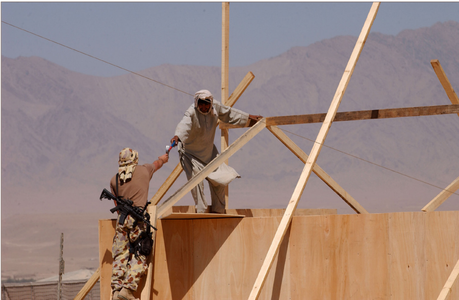
An Australian Combat Engineer assists a locally employed contractor (LEC) on a construction site in a Forward Operating Base in Afghanistan. Photo: Australian Department of Defence, online .
